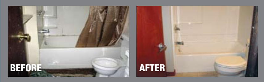
This before and after bathroom remodel shows a kind of home rehabilitation project that would qualify under the Emergency Grant Program and the General Homeowner Rehab Program .
